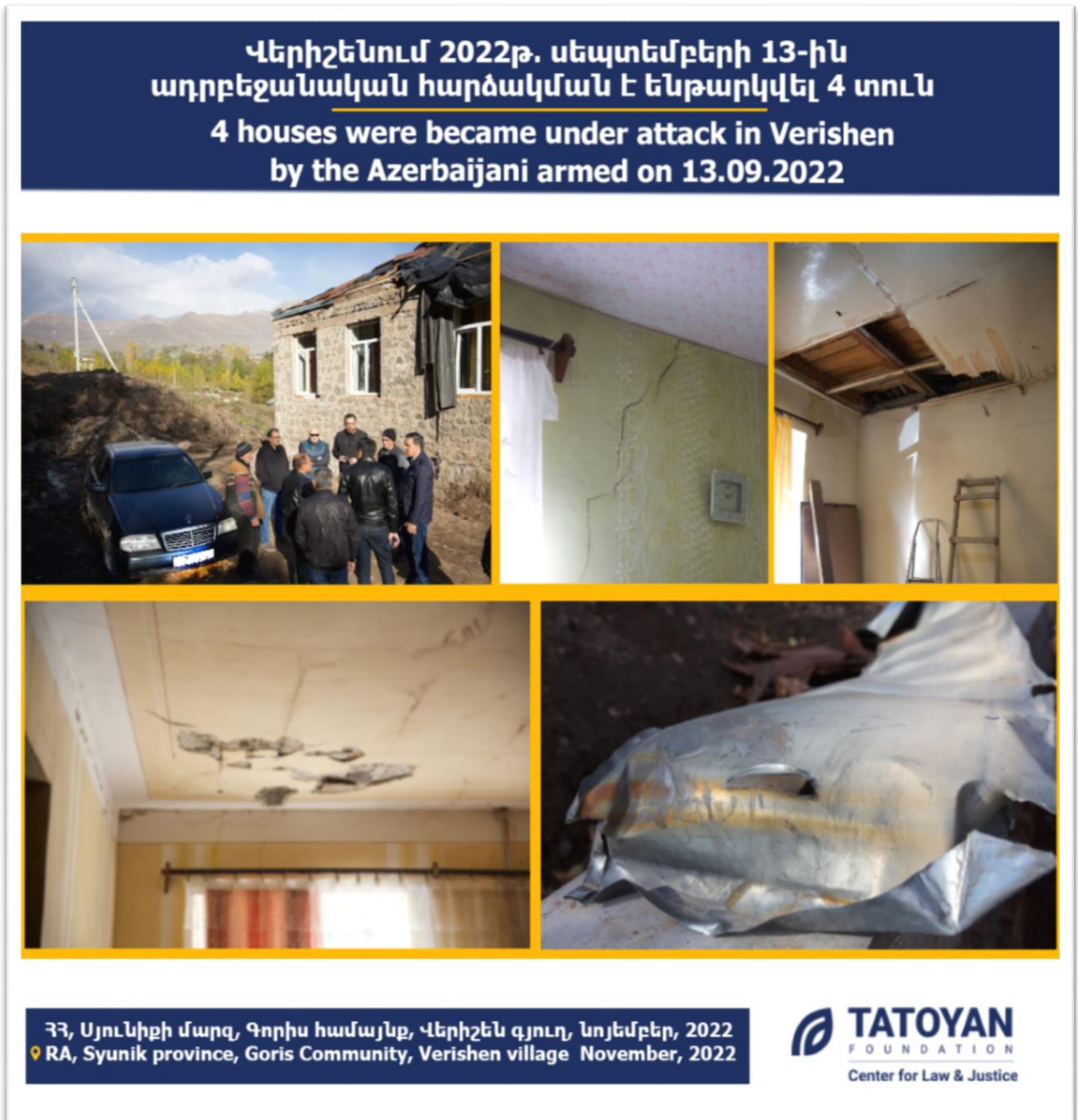
Figure 2: Four houses became under attack in Verishen by the Azerbaijani armed forces in September 13, 2022
